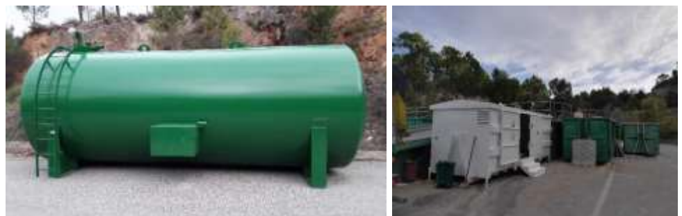
View of the DFCI tank (on the left), view of the DDS (specific waste) bin (on the right)
